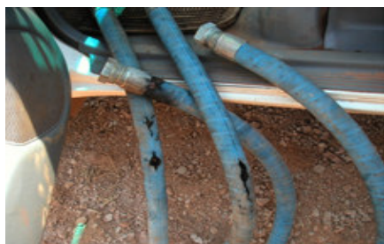
Hoses removed from M41B-870 after the first fire burned through from the inside.
