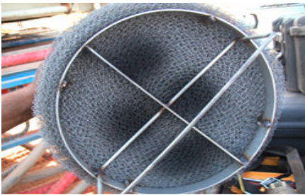
5. Passage of fire up through the new scrubber mesh element into the cylinders.
