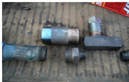
3. The throttle valve and coupling, as well as the inlet to the flowmeter that was at the seat of the fire. There was no significant rise in the temperature at the inlet to the throttle valve at the right of the picture; however, the coupling reached 482 °F.
